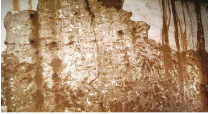
Plate14: Part of an old wall inside Khalwat El-Sayid el-Hassan.
